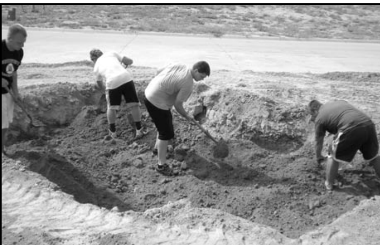
Wayne State College students spent at afternoon recently at the Habitat for Humanity site. Shown here, the students helped pack dirt on what will become the driveway of the new home.
